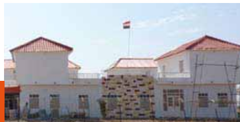
The Professor El Hassan Centre for Tropical Medicine in Doka, Sudan, undergoes major renovation and expansion in 2010.
